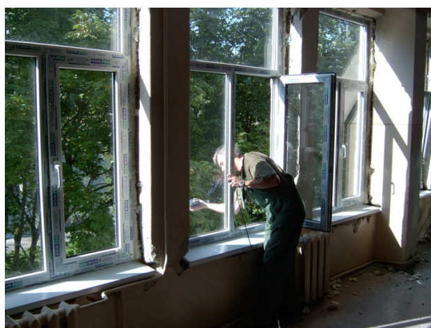
The Project promotes energy efficiency in public sector
